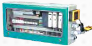
● Elektrik Panosu Electric Panel
