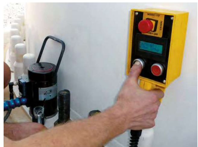
Use of MDS for documentation of bolt pre-tensioning force for tower base bolting of wind power plants.
